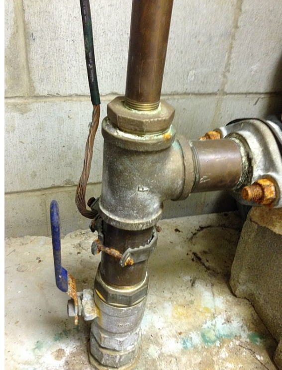
Metal water pipe used as grounding electrode
