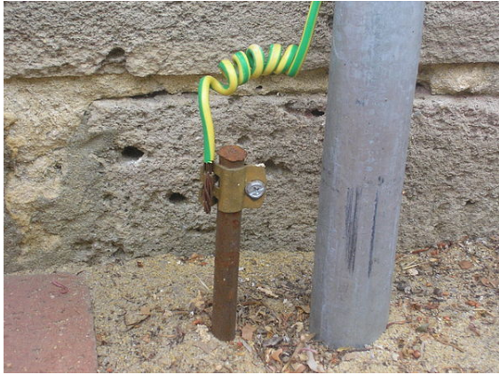
A typical earthing electrode (left of gray pipe), consisting of a conductive rod driven into the ground, at a home in Australia. Most electrical codes specify that the insulation on protective earthing conductors must be a distinctive color (or color combination) not used for any other purpose.
